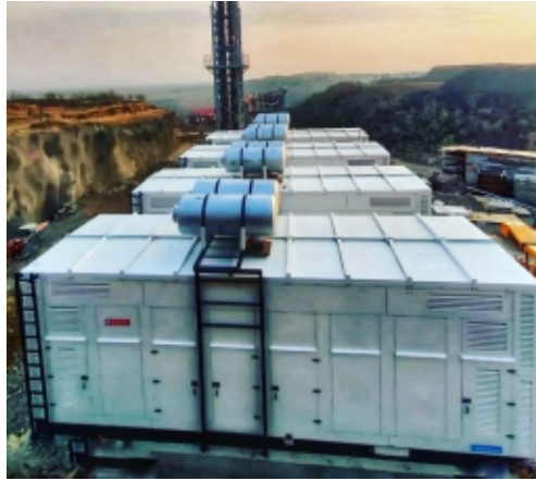
High Speed Roadway Project 2000 kVA x 8
