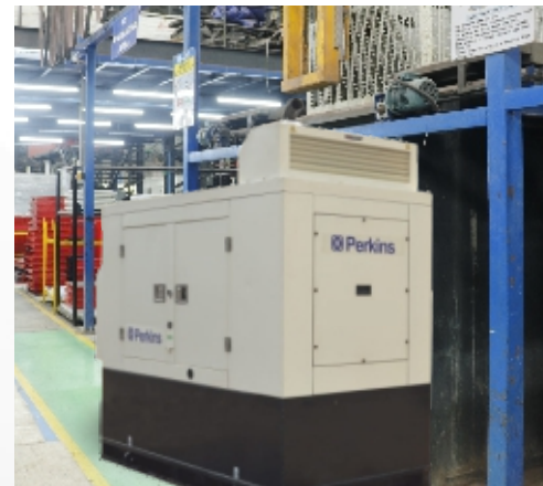
1000 Hours Long Maintenance DG set
