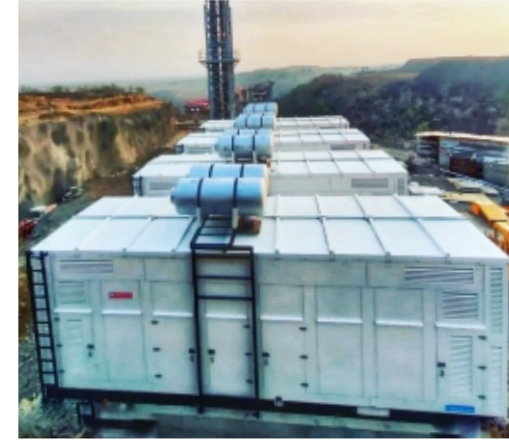
3.3 kV / 6.6 kV / 11 kV High voltage DG set
