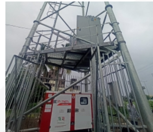
Telecom DG set with Internet Inside
