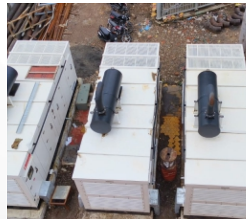
Data Centre Project 750 kVA x 40
