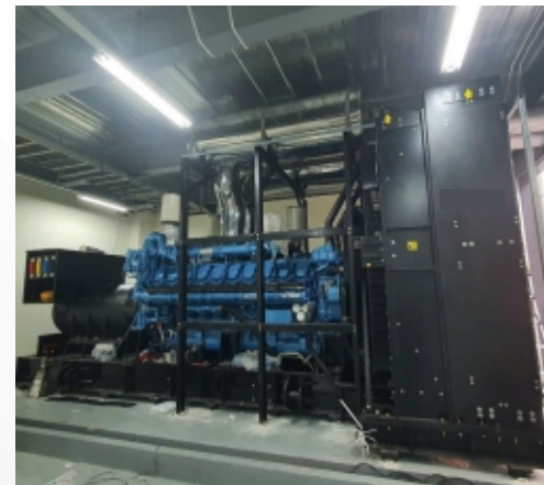
Industrial Unit in Vietnam 2500 kVA x 1
