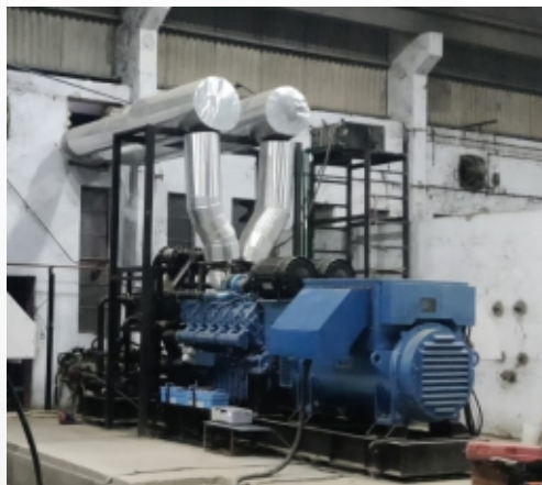
HDPE Manufacturing Units 1250 kVA x 2 & 1010 kVA x 2
