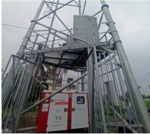
Telecom Towers Across India 10, 20, 30 kVA X40,000
