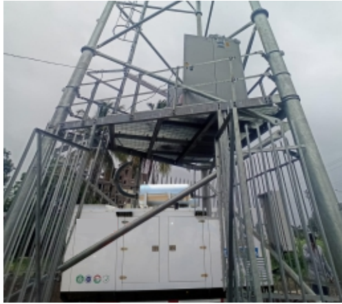
American Tower Company 15, 25 & 40 kVA x 324
