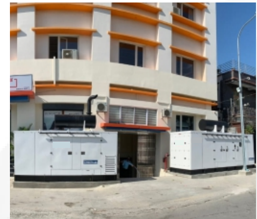
Hospital Project in Myanmar 400 kVA x 2
