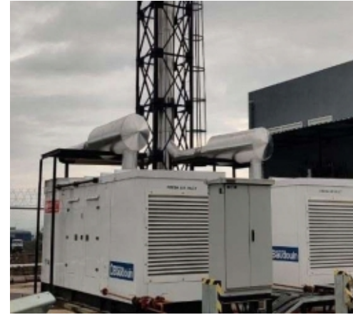
Amazon Project 400 kVA x 2
